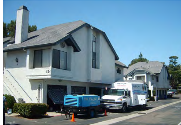
Nu Flow lined all of the hot and cold potable water lines throughout this 190-unit complex.
