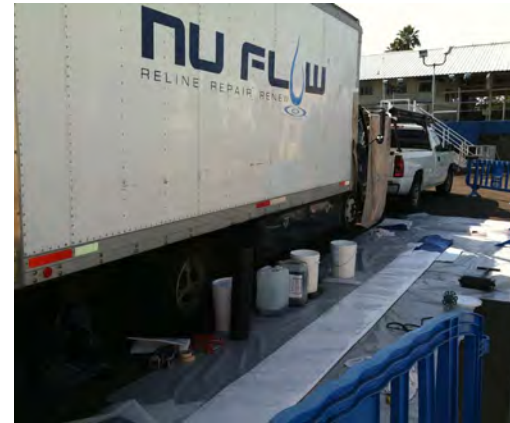
Nu Flow lined a leaking 12"-wide water supply line for a dolphin holding tank that runs 9 feet beneath a concrete sidewalk and landscape at a famous theme park.
