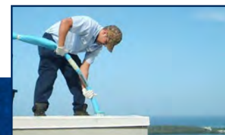
Vertical Sanitary Stacks
