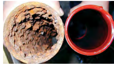
Corroded potable riser and potable riser with Nu Flow's epoxy coating
