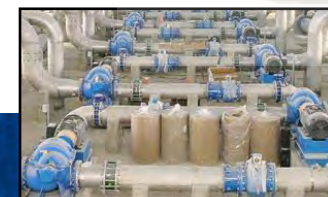
HVAC/Hydronic and Chiller Systems
