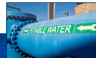
Potable Water Systems
