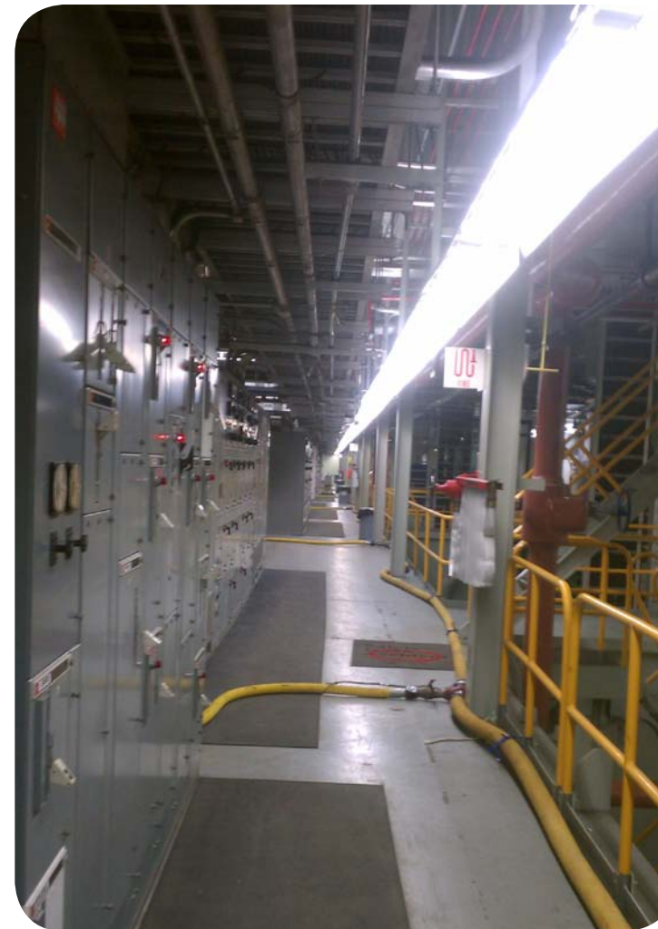
Clean air distribution system hoses used to push the epoxy through this power station's black steel cooling system.
