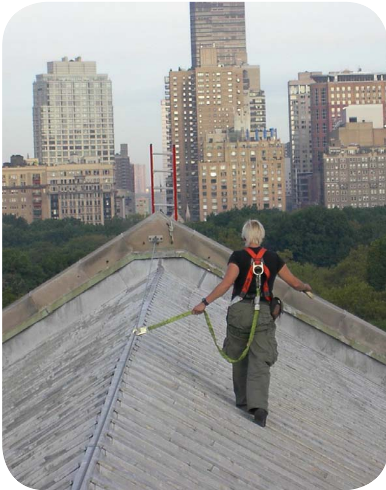
This technician utilized existing access points to rehabilitate this 12-story Synagogue's ten roof drain risers in-place.
